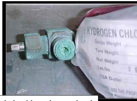
Corroded acid gas lecture bottle
